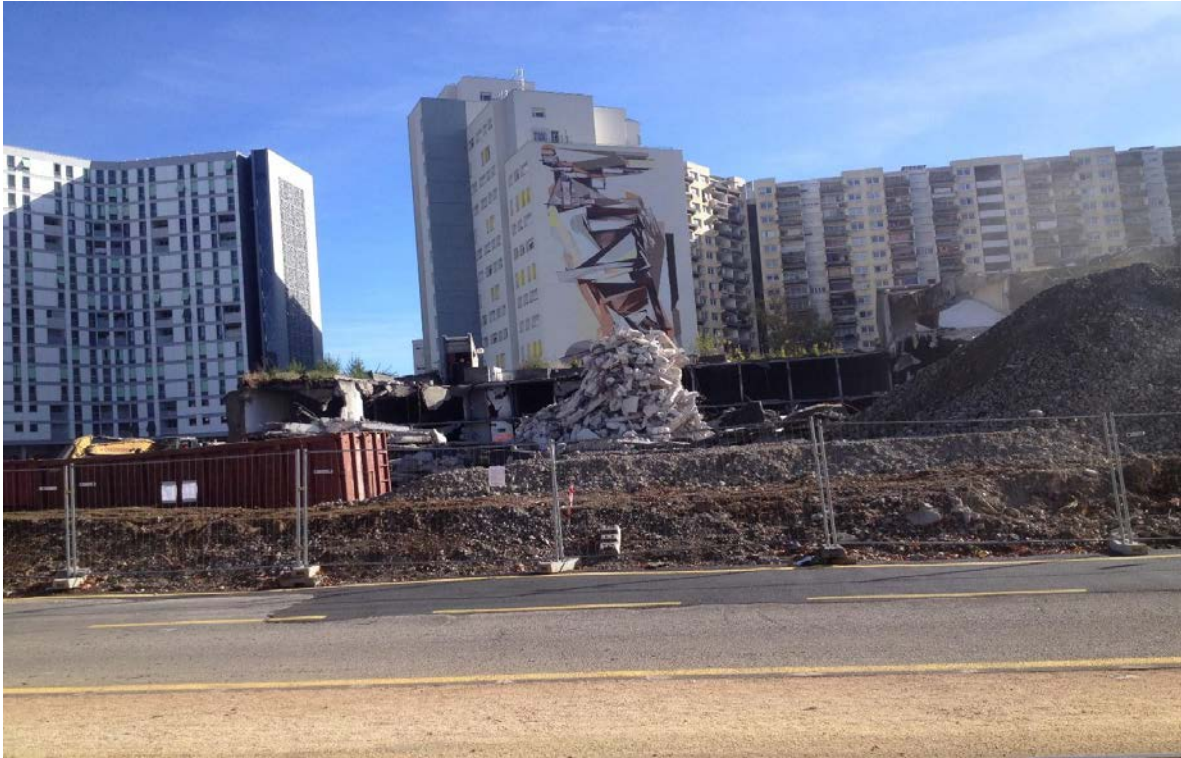
Figure 3.87 “A hole in the wall”, demolition and renovation of the Galerie d’Arlequin. (Photo author 25/10/2017)
