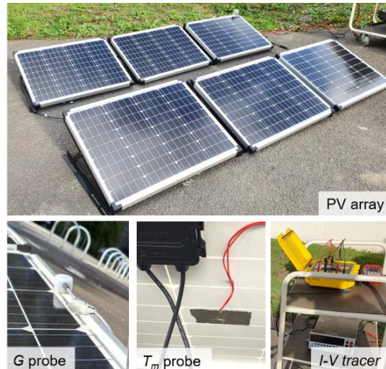
Figure IV-28: Field test setup
