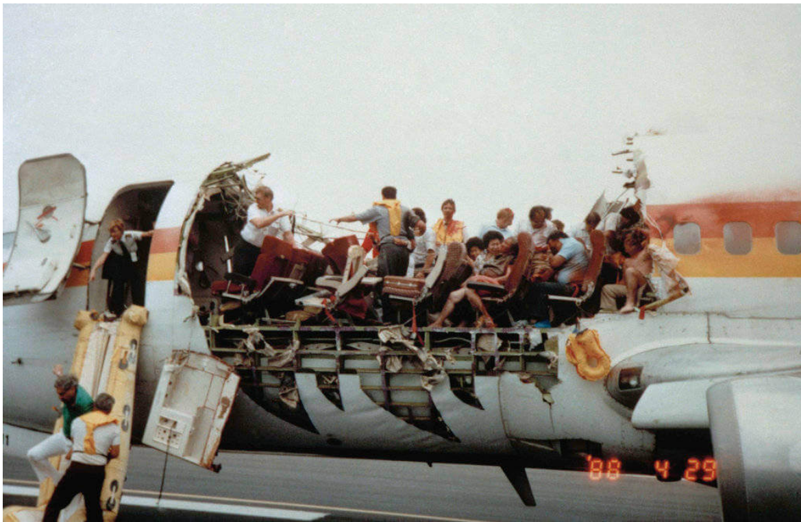
Figure 1-1: Remaining fuselage of Boeing 737-297 of Aloha Airlines Flight 243, after explosive decompression. The NTSB (United States National Transportation Safety Board) investigation report concluded that the accident was caused by metal fatigue exacerbated by crevice corrosion (Source: Wikipedia)
