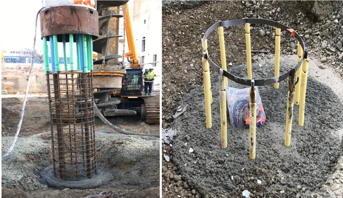
Figure 2.23 Installation of the reinforcing cage in the wet concrete using a vibrator
