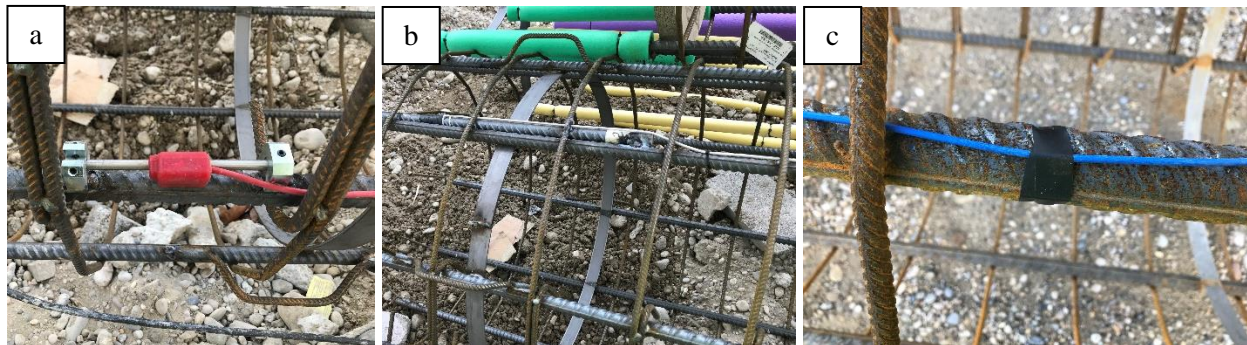
Figure 2.20 Installed examples of (a) VWSGs, (b) ERSGs and (c) Optical fibers
