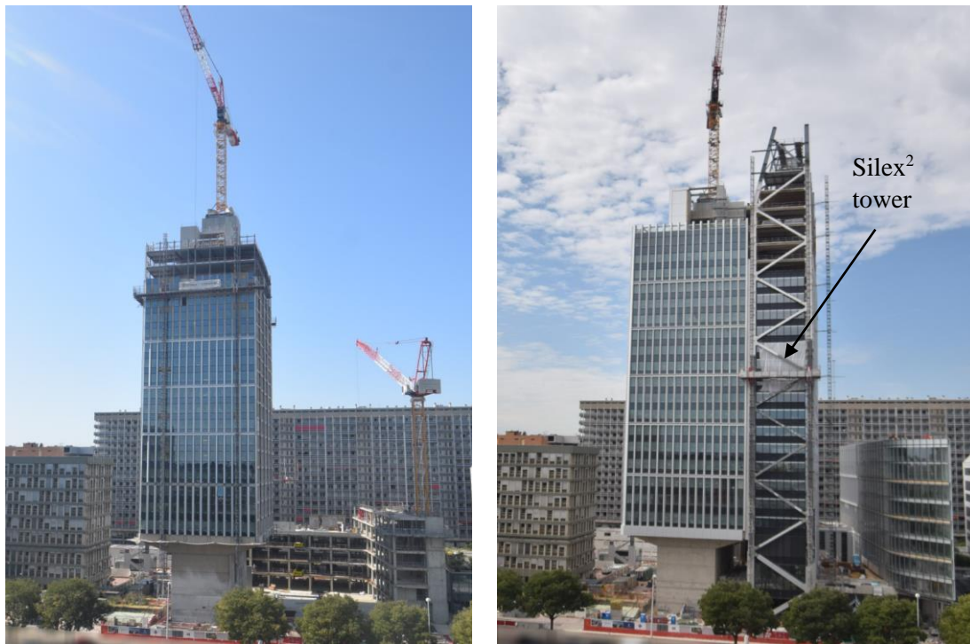
Figure 4.7 Pictures of the construction site in September 2019 and September 2020 (at level R+25)
