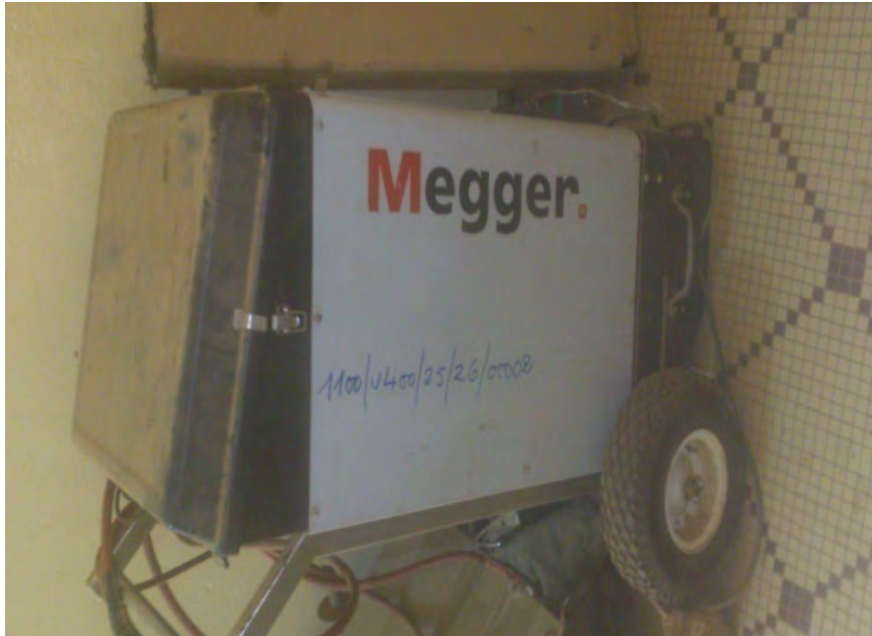
Photo 36 : Power Fault Locator, PFL 40 A Source : Abdourazack N. A., 2018
