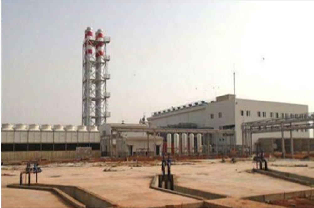
Photo 31: Centrale diesel de Gorou Banda, 2018
