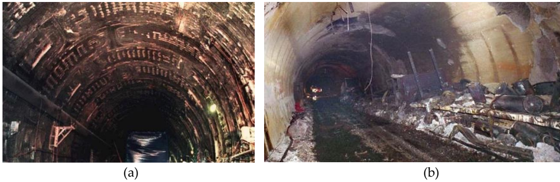
Figure 3.17 After fire: a) tunnel under La Manche in 1996 [32], b) tunnel Mont Blanc [33].
