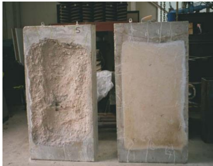
Figure 3.22 Efficiency of polypropylene fibers against spalling due to fire. On the left: a sample without fibers, on the right: a sample with polypropylene fibers [52].
