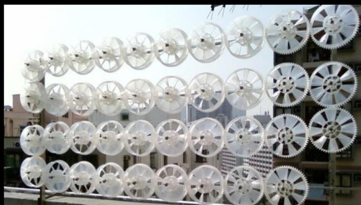
The first micro-turbine array set up in Hong Kong. It includes 40 turbines, which has daily production capacity of $60Wh with average wind speeds of 5.5 m/s. This installation was made in November, 2006, and is large enough to power all of the lights in the apartment below. If space is available, it is suggested to spread these turbines along a single row, instead of four rows. This is because the anchoring with the posts will be easier and more secure. The taller the display is, the stronger the posts and anchoring system needs to be.
