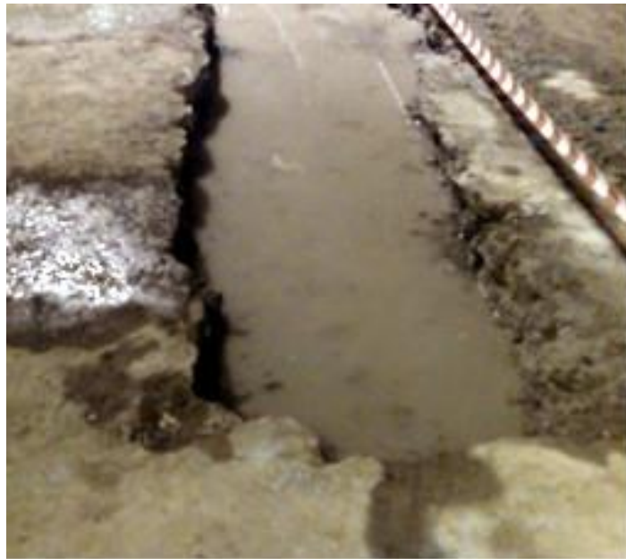
Figure 2.17. Water in the area of local dismantling of the rigid base and leveling layer
