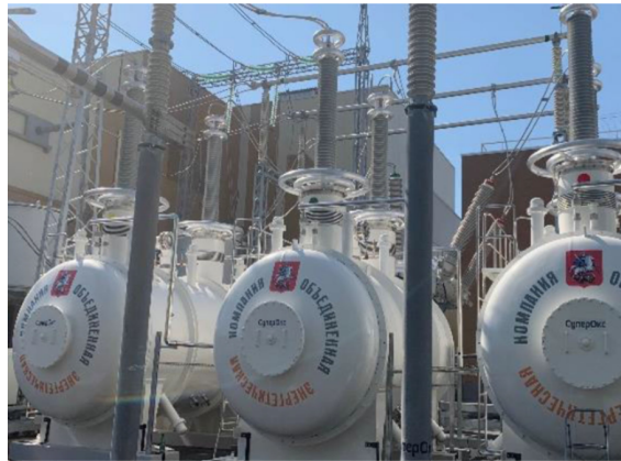
Figure 1.23: Picture of the 220 kV R-SFCL at the substation in Moscow, from [6].
