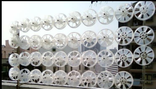
The first micro-turbine array set up in Hong Kong. It includes 40 turbines, which has daily production capacity of $60Wh with average wind speeds of 5.5 m/s. This installation was made in November, 2006, and is large enough to power all of the lights in the apartment below. If space is available, it is suggested to spread these turbines along a single row, instead of four rows. This is because the anchoring with the posts will be easier and more secure. The taller the display is, the stronger the posts and anchoring system needs to be.
