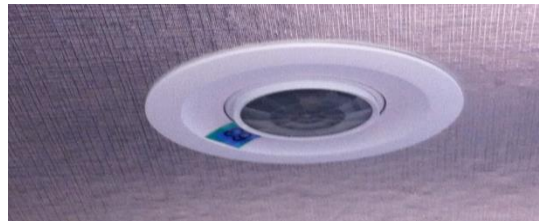
Figure 18. Luminance and presence sensor
