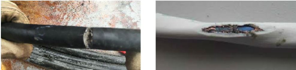
Figure 1.7: Hard (left image [source]) and soft (right image [source]) faults appearing in wiring networks.
