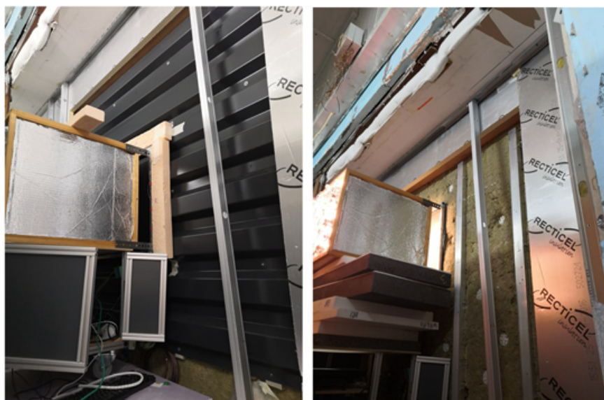
Figure 5.18: Prototype setup on (left) the metal cladding and (right) the external surface of insulation layer of the EWI wall.
