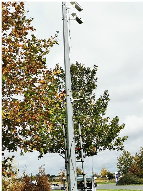
Figure 5.9: An intelligent camera installed on a road pole close to the roundabout test-bed in Rambouillet. In order to obtain the best detection performance, we tested two different models of cameras that are visible on the pole.
