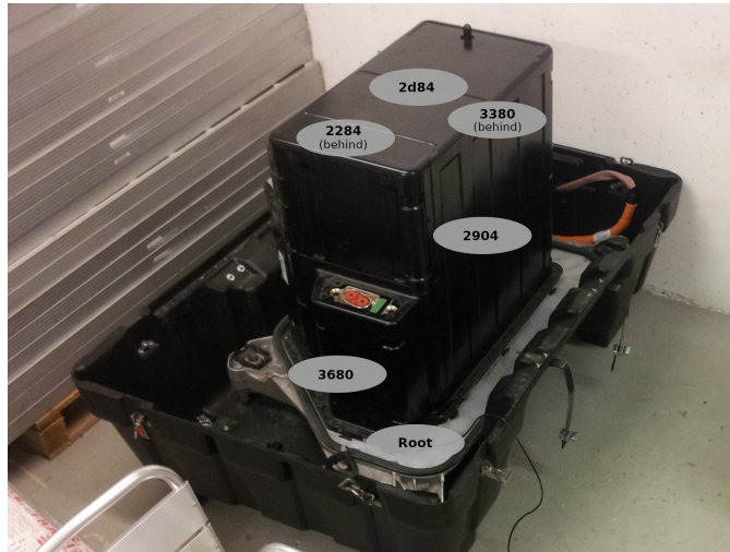
Figure 3.30: Measuring link quality inside a Fluence pack with Wi-Fi interference: motes layout
