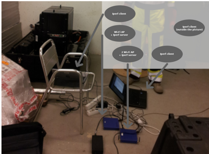
Figure 3.29: Link quality measurement inside the Fluence battery pack with continuous Wi-Fi communication in the environment using the IPerf software.
