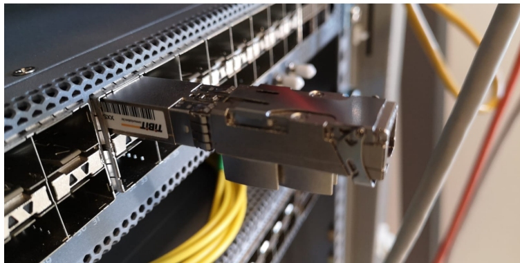
FIGURE 6.4: XGS PON's mini OLT plugged on a switch
