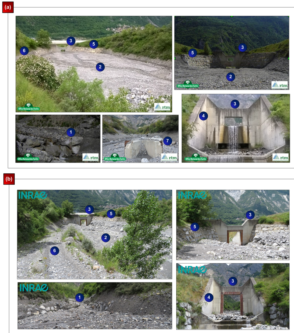
Figure 6.2: Claret retention system showing the old and the new design of the retention dam: (a) old design ©ONF-RTM/S. Carladou 23/05/2018; (b) new design ©INRAE/J.-M. Tacnet 05/07/2021. (1) upstream inlet check dam (2) retention basin, (3) retention dam, (4) downstream counter dam, (5) lateral dykes, (6) access track and (7) debris flow breaker.
