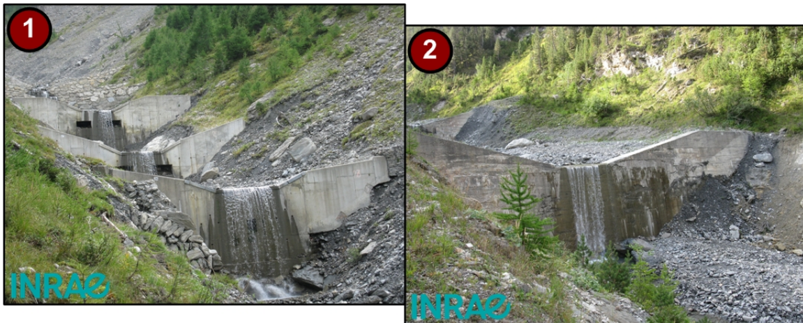
Figure 1.11: Torrent check dams: (a) Check dams series; (b) Single check dam. Saint Antoine torrent, France, 2014. Source: ©INRAE/ETNA.
