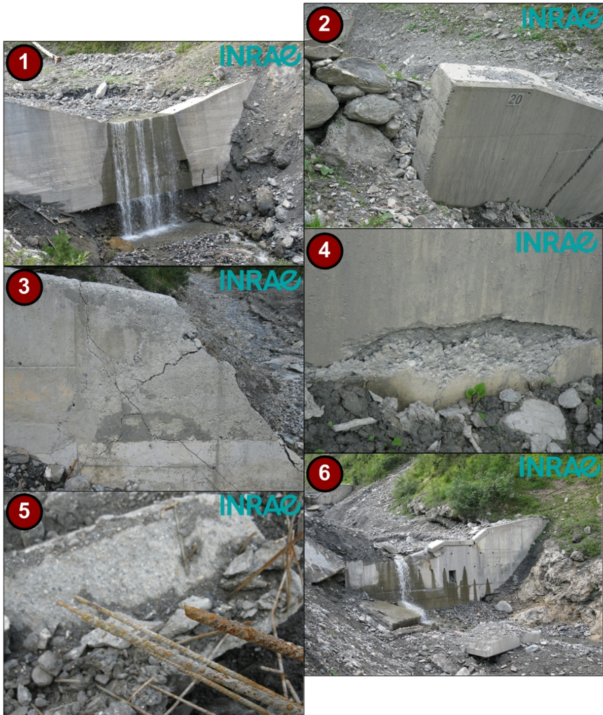
Figure 1.17: Examples on the types of functional and structural failures check dams may be subjected to: (1) scouring under dam's foundation; (2) erosion of banks due to lateral bypass; (3) presence of cracks; (4) concrete corrosion; (5) steel corrosion; (6) total destruction. Saint Antoine torrent, France, 2014. Source: ©INRAE/ETNA.
