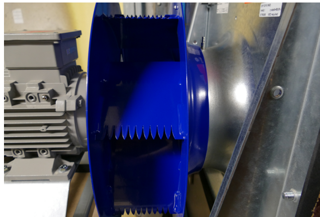
Figure 1.45 – Impeller with trailing-edge serrations mounted on the shaft
