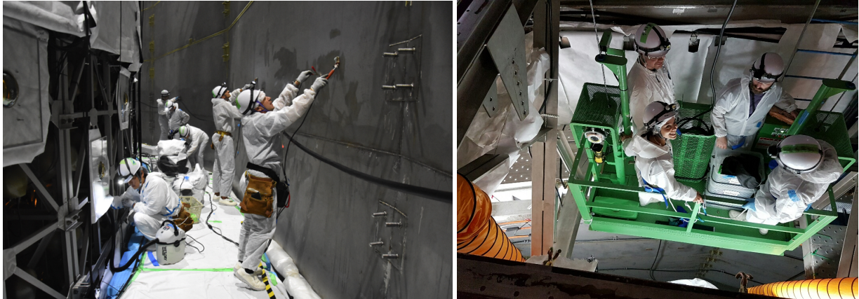
FIGURE 3.2: Pictures taken during refurbishment work. Left: OD repair works on the wall barrel and Tyvek sheets replacement performed every day on a floating platform. Right: gondola to reach water level.
