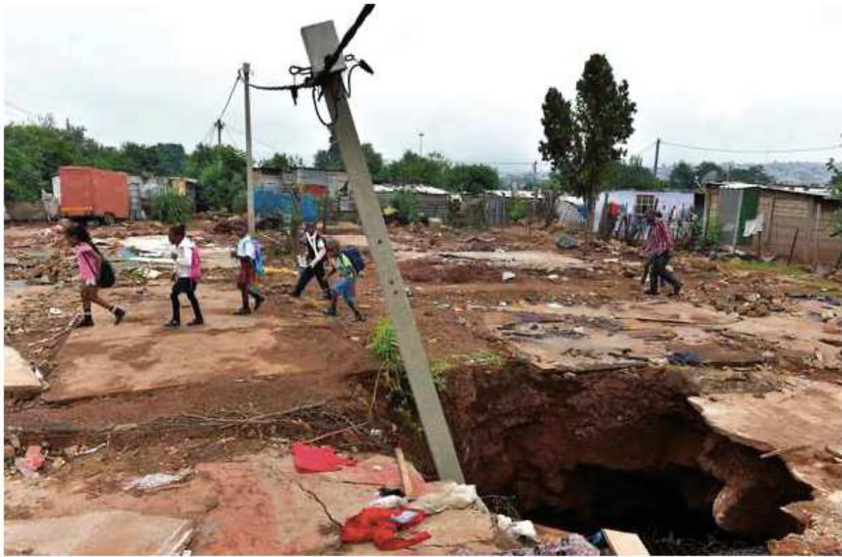
Children walk past a sinkhole where a number of shacks were damaged in Jeffsville informal settlement in Atteridgeville. Picture: Oupa Mokoena
