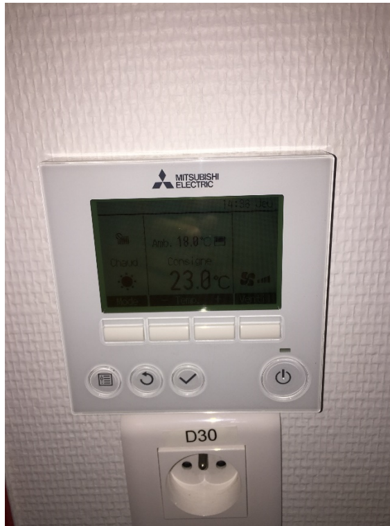
FIGURE 4.7: HMI installed in each room of the building.
