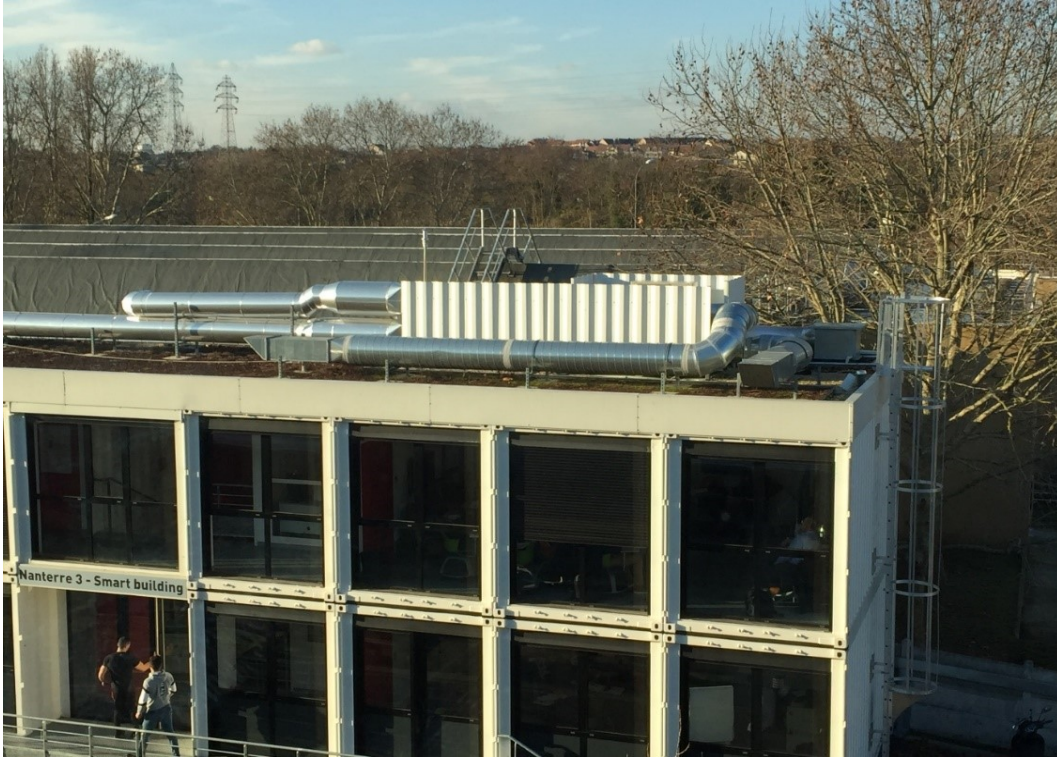
FIGURE 4.6: Installed weather station and VRF system heat pump setup on the building.
