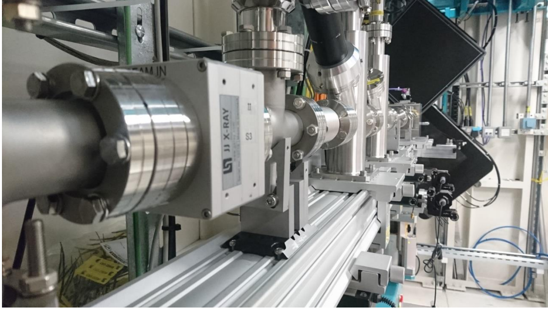
Figure III. 3 View inside I15-1 Experimental Hutch.
