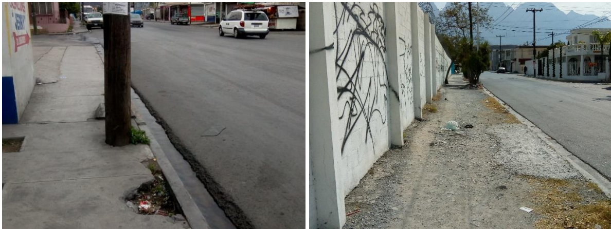
Figure 84 Deteriorated sidewalks on Loma Linda.
