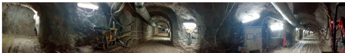
Figure 1.7 – 360° view from the cavity common to both galleries during the drilling works.
