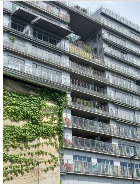
Figure 123 E5 building, Fault, south façade. Source M. Apostolou
