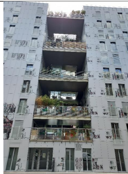
Figure 132 E5 building, fault, north façade. Source M. Apostolou
