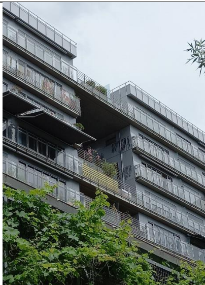
Figure 131 E5 building, fault, south façade. Source M. Apostolou
