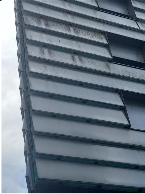
Figure 66 The inclined panels, spaced at approximately 150 mm intervals are attached to a concrete support insulated with several layers of insulation in order to reach the environmental objectives of the objectives of the project (Climate Plan of the City of Paris) and obtain the BBC label. Source M. Apostolou
