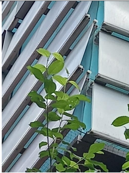
Figure 67 detail of the inclined panels of the façade of the E1 building. Source M. Apostolou
