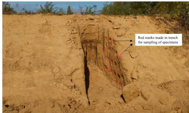
Fig. 3-1 Trench excavated in the lime-treated embankment (T2) for the sampling of specimens.
