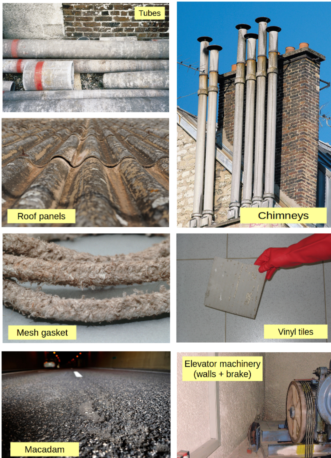
Figure 1.2: Presence of asbestos contamination inside residence-B
