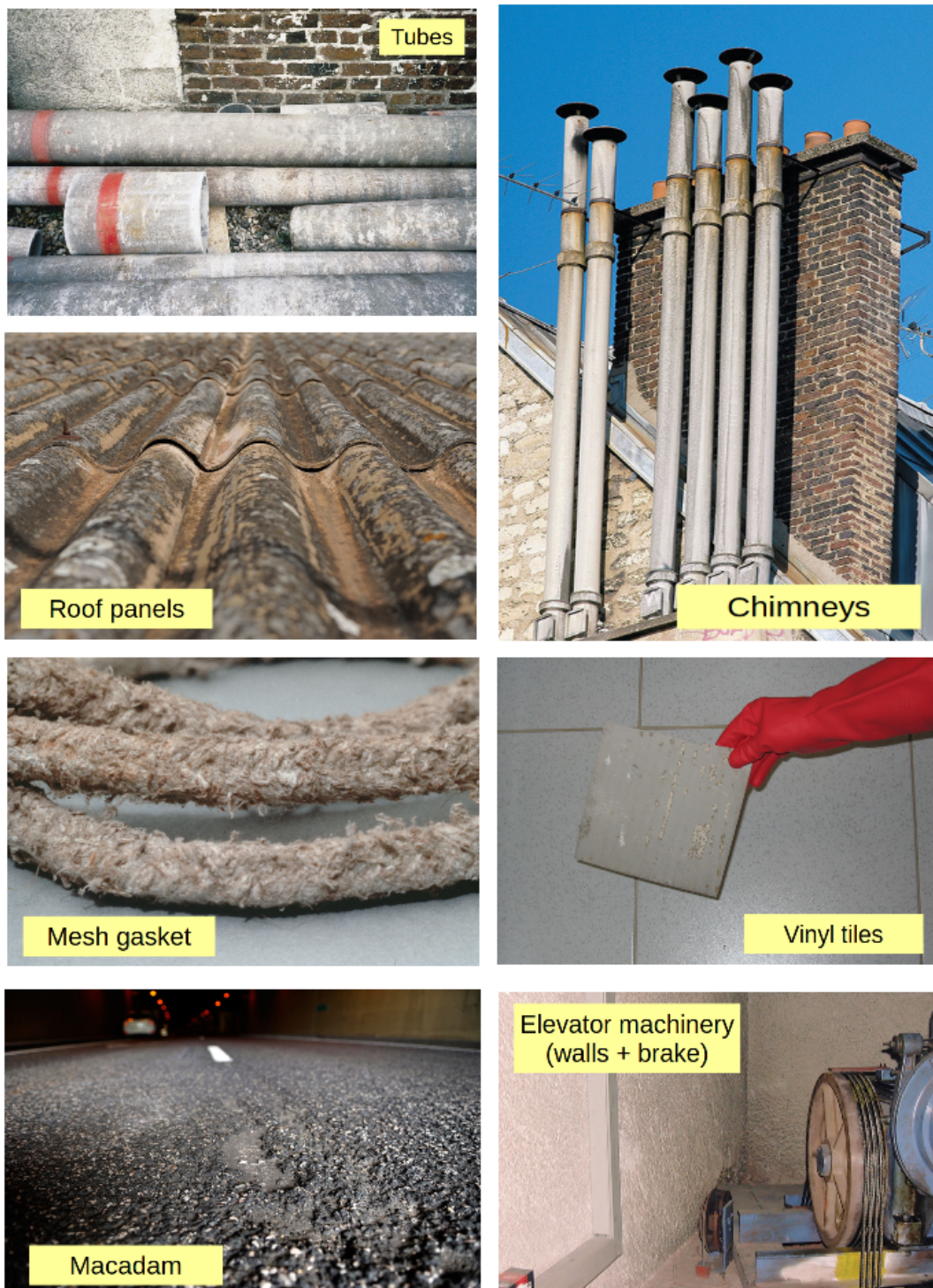
Figure 1.2: Presence of asbestos contamination inside residence-B
