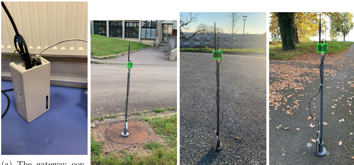
(a) The gateway connected to the antenna cable. (b) The end node at location 4. (c) The end node at location 5. (d) The end node at location 7.
