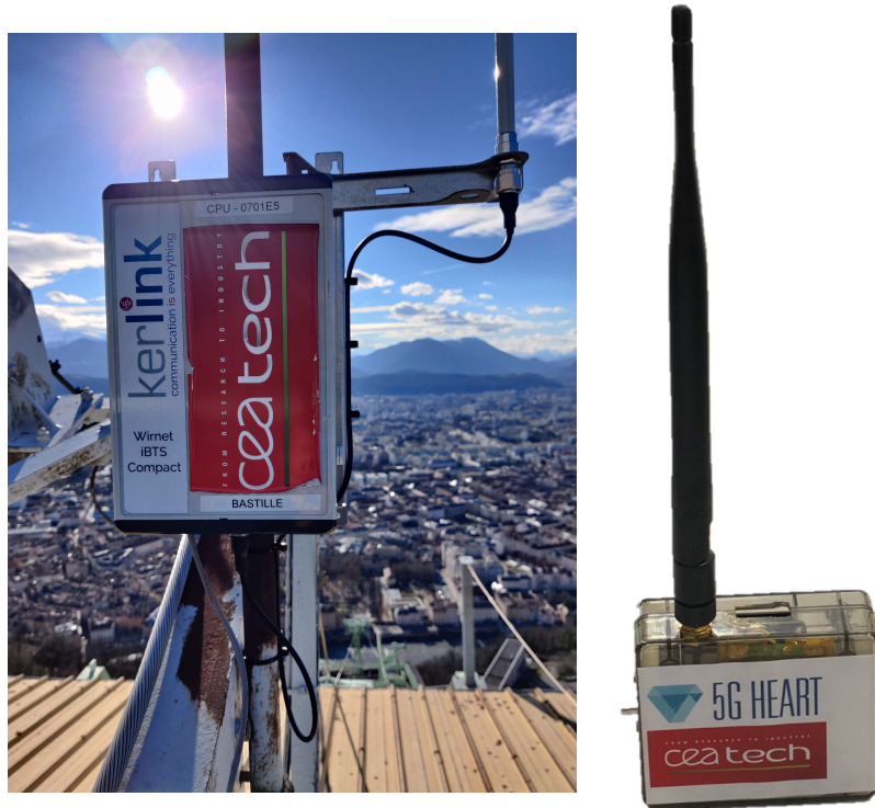
(a) Gateway BS_3 which is installed on the roof near the cable car station at Bastille, (b) Tag which was used to collect the data Grenoble
