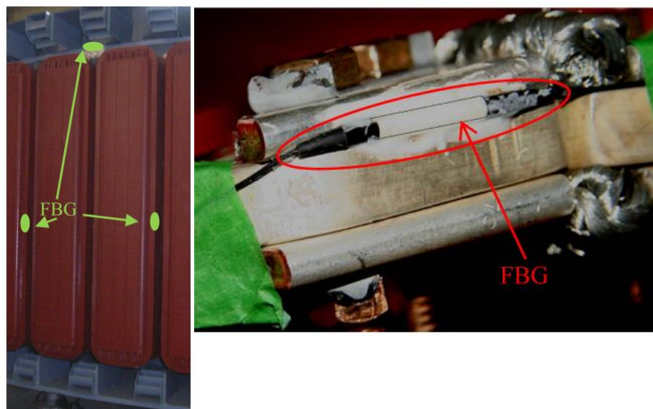
Figure 25: Fans and poles of the unit under investigation (left) and FBG sensor installed on a pole-to-pole connection (right)
