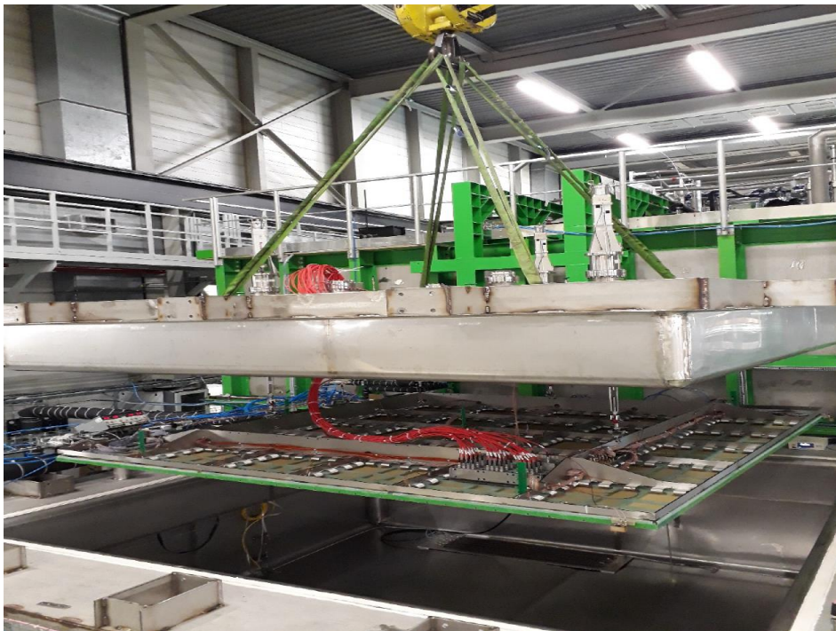
Figure 3.16: Closing of the coldbox with a mounted CRP
