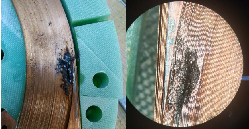
Fig. 122. Melting of the conductor on several turns due to a short circuit causing a hole in the winding.
