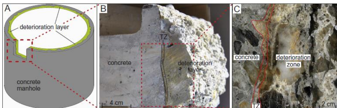
Figure I-11. A scheme of a manhole and the sampling cut with a clear view of the transition zone (TZ) [48]
