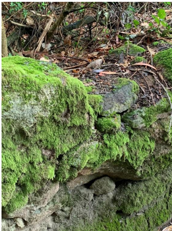
Figure 82 - Wall covered on moss
