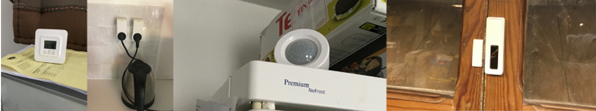
Figure 4.3 – The positioning of PIR sensors, power sensors, contact sensors and some of their images in Cestas site
