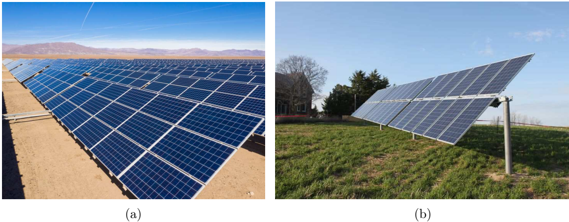
Figure 1.3: (a) A fixed-tilt flat plan PV plant [4], (b) a single-axis tracking plant [5].
