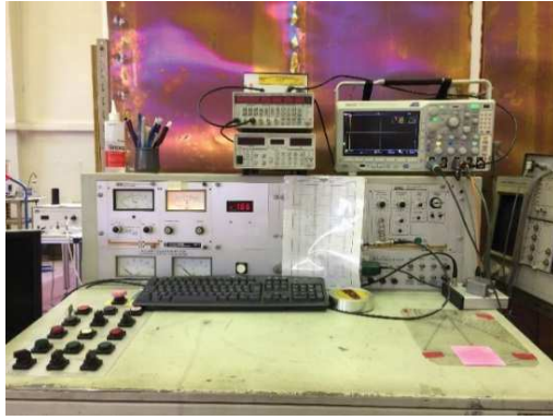
Fig. 5: Control desk of Marx generator.
