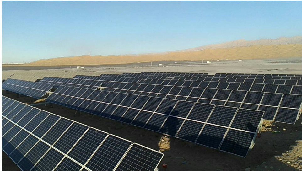
(a) Photograph of the PV tracking system installed at Wuhai, China. Photograph courtesy of Canadian Solar
