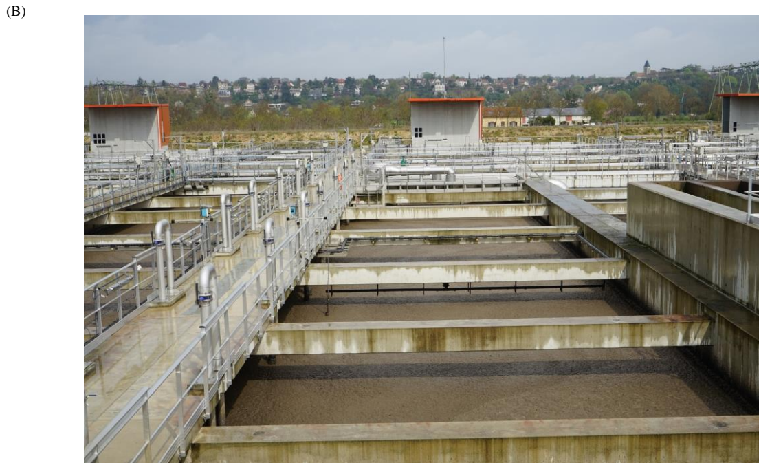
Figure 2.7: Schematic representation of SAV-MBR (A) and photo of anoxic zone from one of the biological basins (B).
