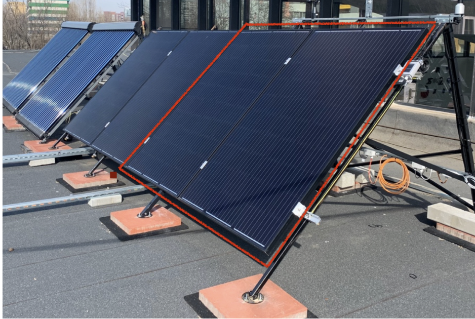
FIGURE 5.10: Photography of the photovoltaic panels installed on the roof
