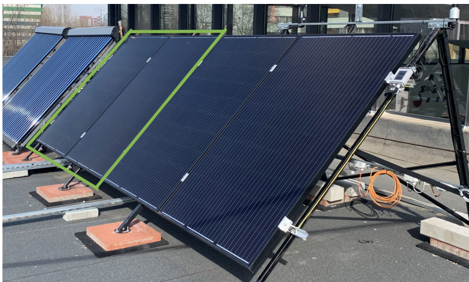
FIGURE 5.13: Photography of the PVT panels installed on the roof
