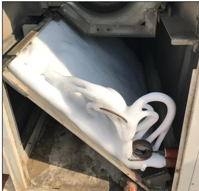
Figure 5.2. Ice formation on HVAC evaporator unit due to improper maintenance & dust accumulation
