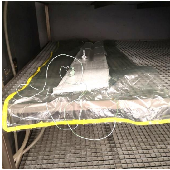
Fig. 2. 9. Structure covered with vacuum bag and prepared for polymerisation in the oven
