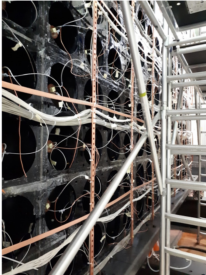
Figure 2.9 – Side view of a main calorimeter wall. Visible are the optical fibers, electric cables and signal cables, which deliver the high voltage and retrieve the PMT signals.
