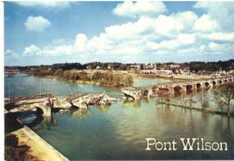
Figure 1.3: An example of a bridge collapse due to scour erosion at the foundations: Loire River, Tours, 1978.
