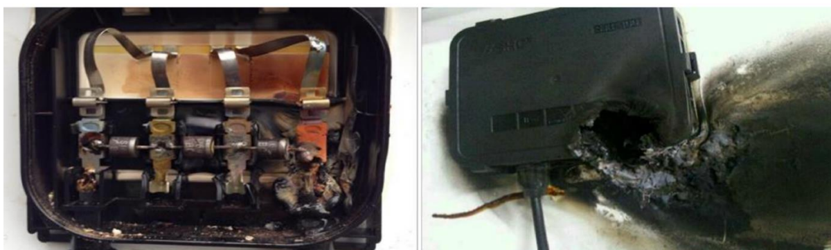
Fig.III.10: Junction box failure [14]
