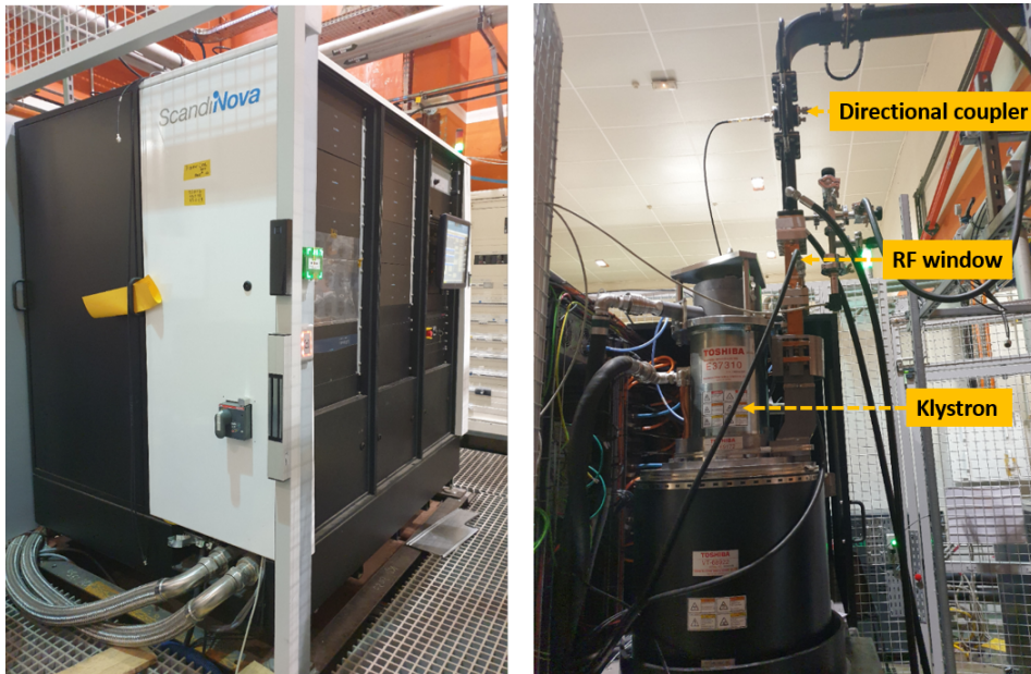
Figure 2.9: Installation of the ThomX RF source (ScandiNova modulator K2-2 & TOSHIBA Klystron E 37310).
