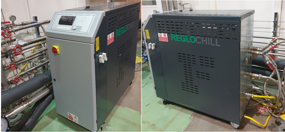
Figure 2.44: Picture of the Regloplas temperature control systems.
