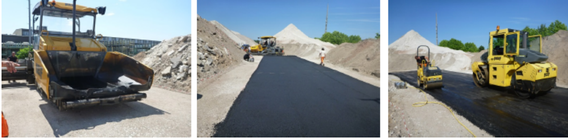
Figure III.1.3: Construction of lower layer: Finisher on unbound granular base course, test surface, compaction of the surface
