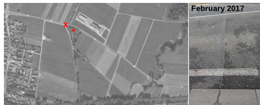
Figure IV.1.15: RD4: Crack between the section built in on 29/10/15 and the section built on 30/10/15
