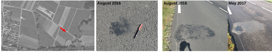
Figure IV.1.11: RD4: Medium and big bitumen accumulations
