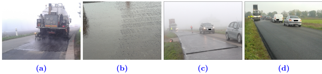
Figure IV.1.9: RD4 maintenance works: Construction steps: (a): Emulsion sprayer at the beginning of the construction works; (b): Difference in emulsion application rate, left: section N1, right: section Ref 6 cm; (c) Application of grid 5 in the curve (d) Finished road
