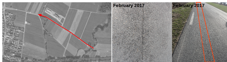
Figure IV.1.14: RD4: Superficial, very straight crack
