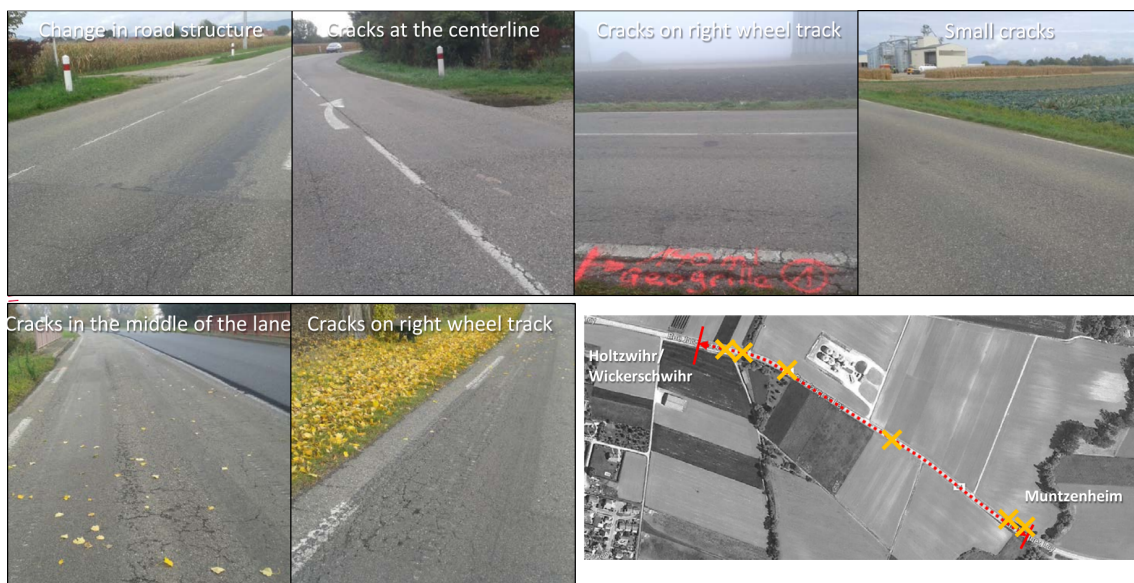
Figure IV.1.4: Photographs of the RD4 before maintenance and location of the pictures taken (map on the right, second line)
