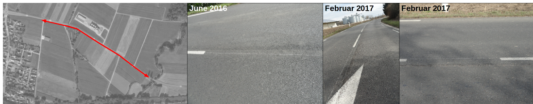
Figure IV.1.12: RD4: Crack at the centre line
