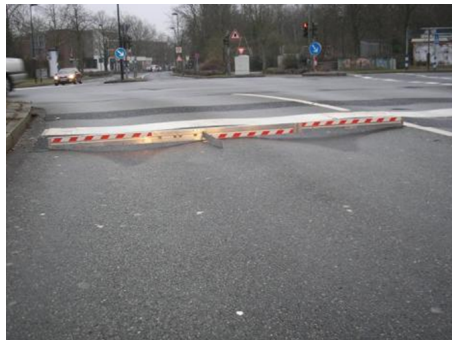
Figure I.1.4: Ruts on a road [AP9 15]
